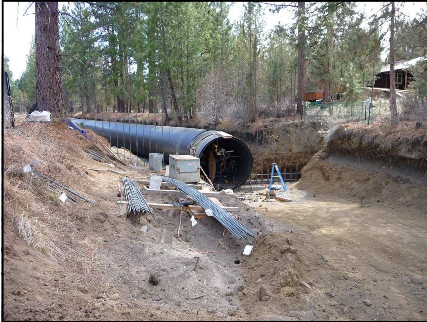
Tumalo Irrigation District in the Deschutes River Basin is replacing over 6 miles of open canal sections with large diameter conduit . This latest phase of construction will save over 530 acre-feet of water once lost to seepage.
